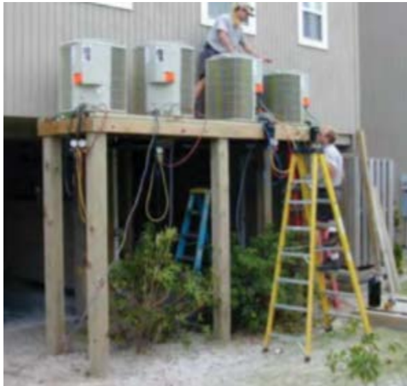
Figure 3.25 – Two workers elevate condenser units on a platform above BFE (Image courtesy of FEMA)
