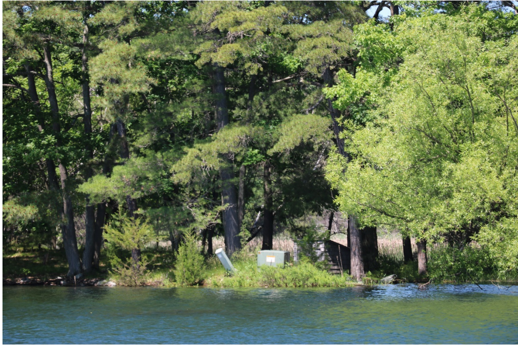
Figure 2.58 – A generator sits on the shoreline, just feet away from high water
