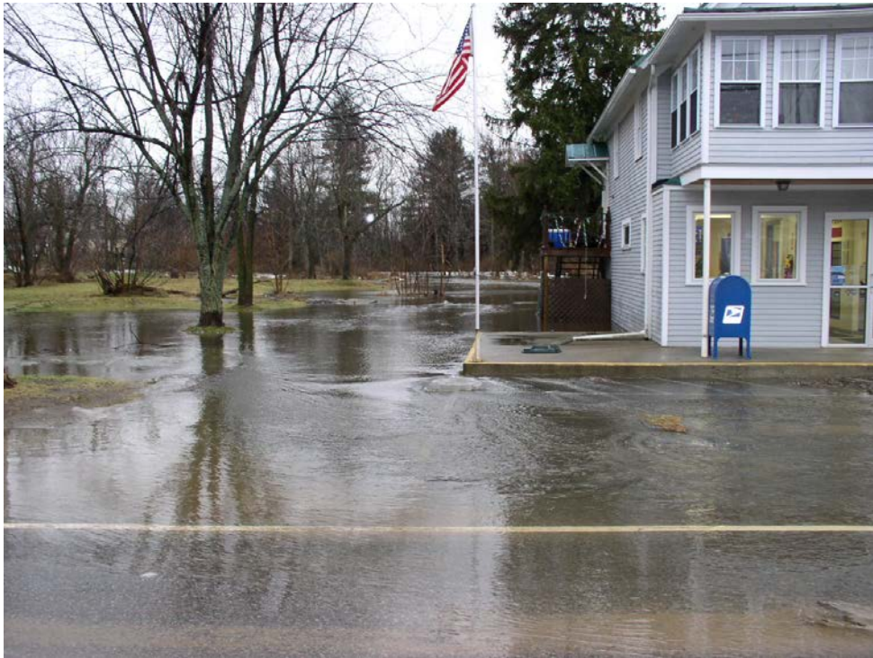
Figure 2.43 - Buildings in the Town of Hammond, Hamlet of Chippewa Bay, are inundated by flood water. This can lead to flooded basements, loss of property, and physical damage to concrete foundations over time
