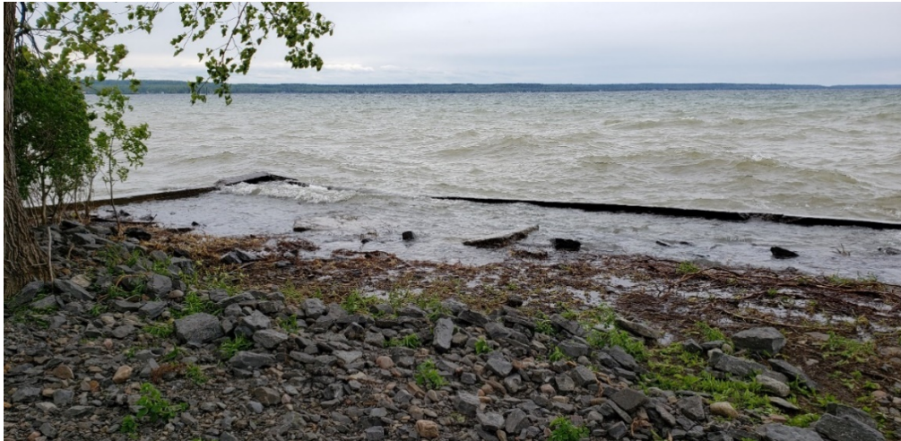
Figure 3.24 – A concrete seawall less than 50 years old becoming ineffective, due to changing conditions and limitations of material properties in design
