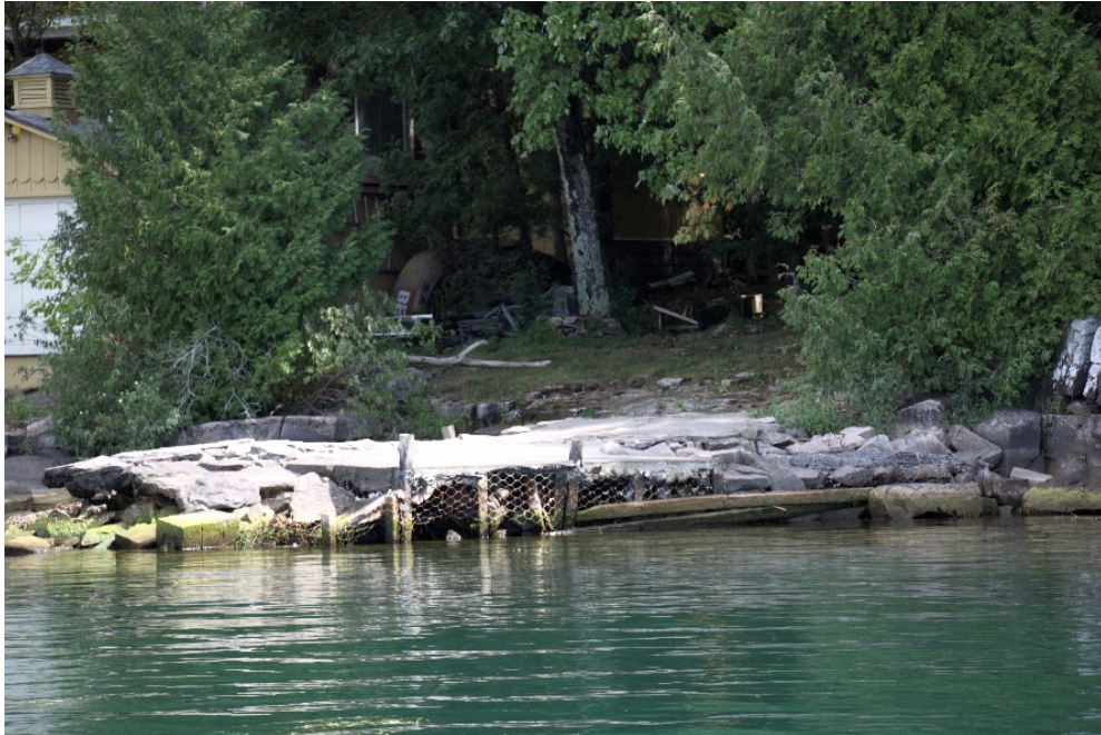
Figure 2.44 – A residential dock crumbles
