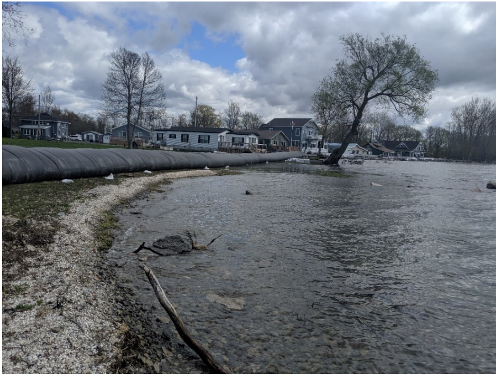
Figure 3.22 – Emergency response measures (e.g., Aquadam and supersack installation) may be warranted to protect properties that are not resilient
