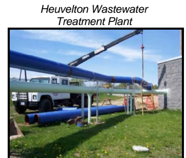
Heuvelton Wastewater Treatment Plant Photo Courtesy of the St. Lawrence County Planning Office
